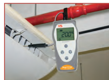
Temperature measurement in air conditioning system
